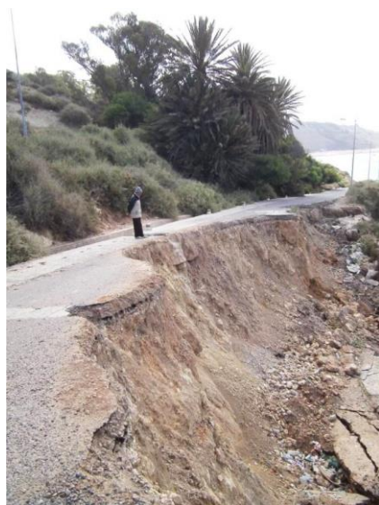
Figure 5: Road near Safi prone to landslide
